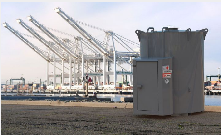
12,500 LITRE VERTICAL BULK DIESEL TANK
